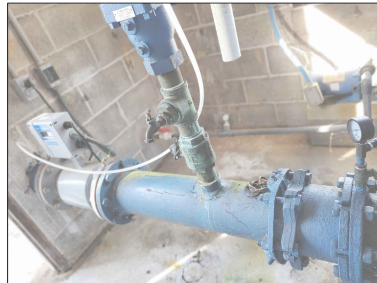
PHOTO 4 - LOOKING NORTH TOWARD WELL DISCHARGE
