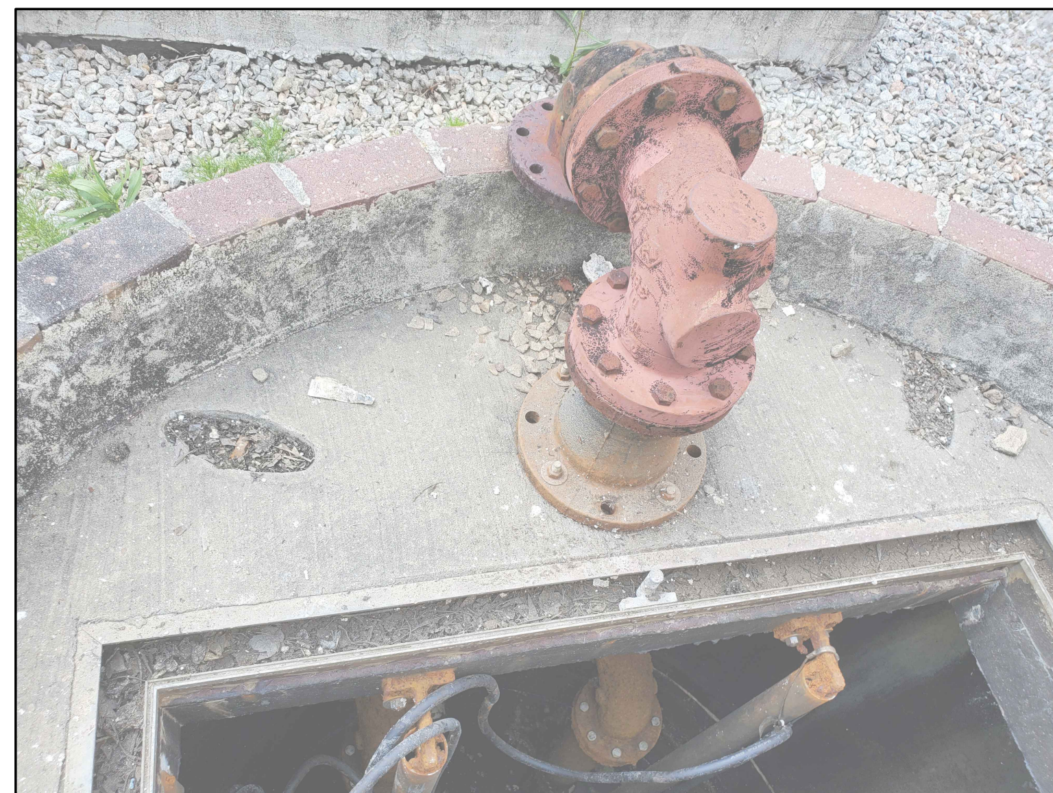
PHOTO-9 LOOKING NORTHWEST AT WET WELL
