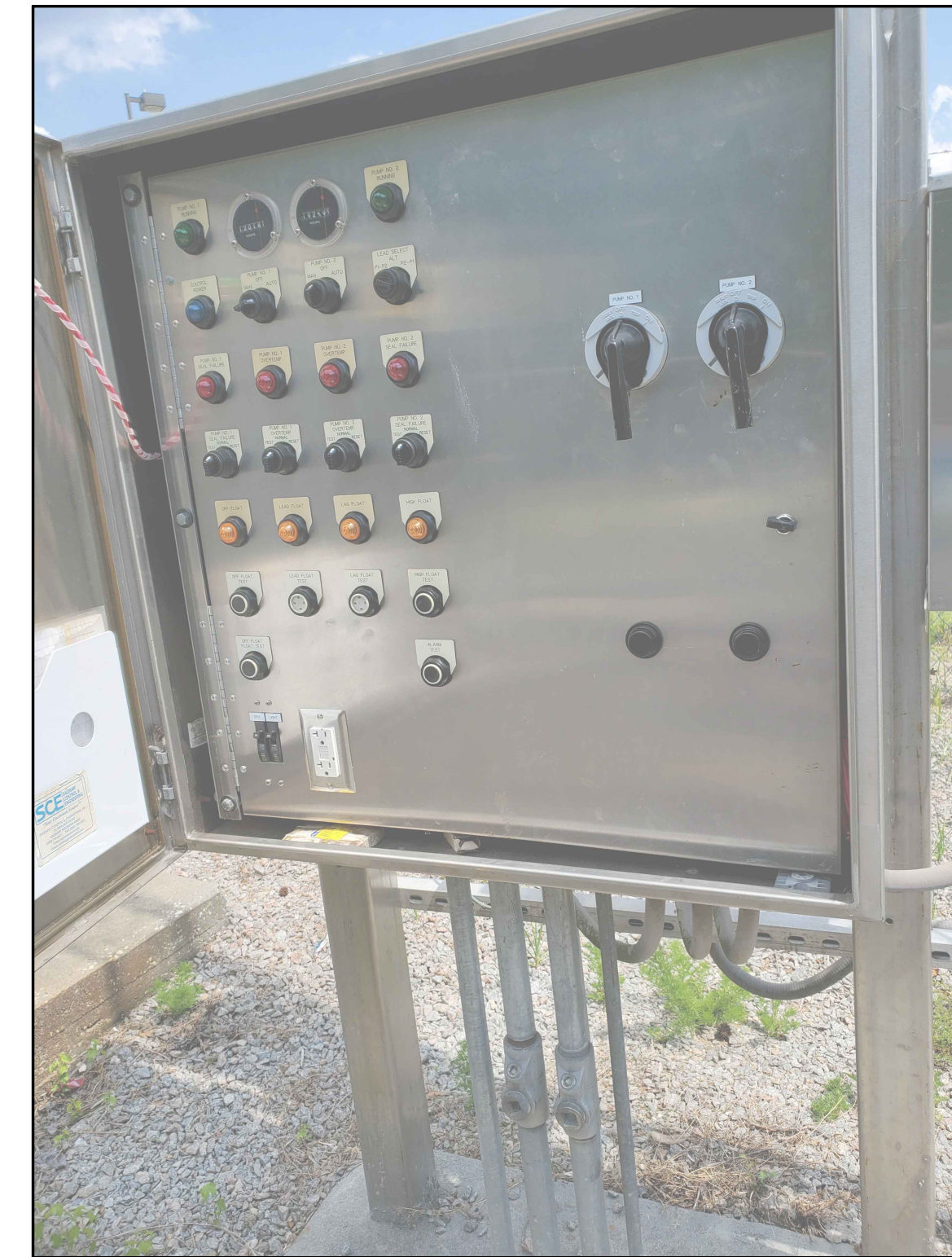
PHOTO-10 LOOKING SOUTH AT PUMP STATION CONTROL PANEL
