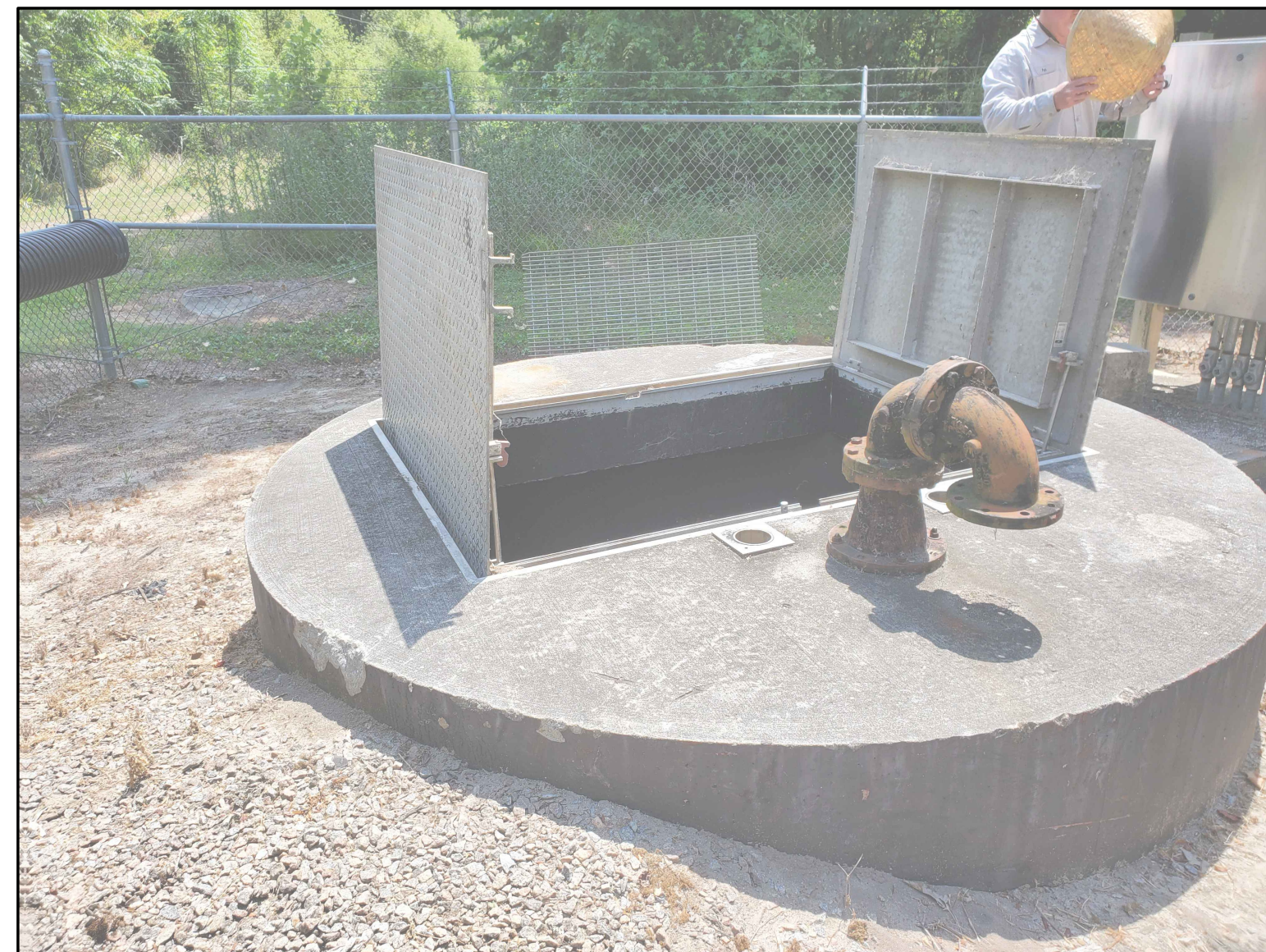
PHOTO-5 LOOKING SOUTHEAST AT WET WELL
