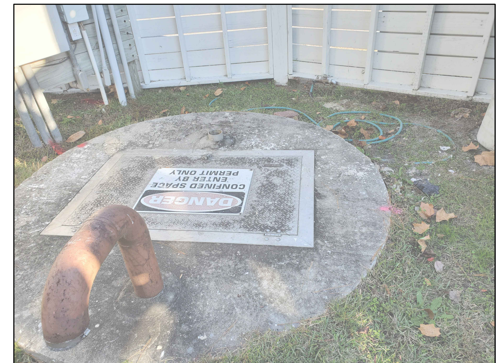
PHOTO-6 LOOKING EAST AT WET WELL
