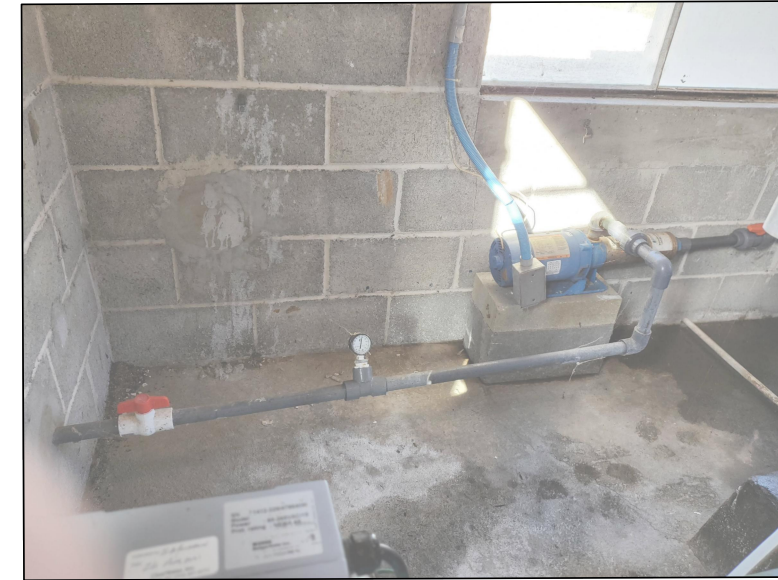
PHOTO 5 - LOOKING NORTH TOWARD BOOSTER PUMP
