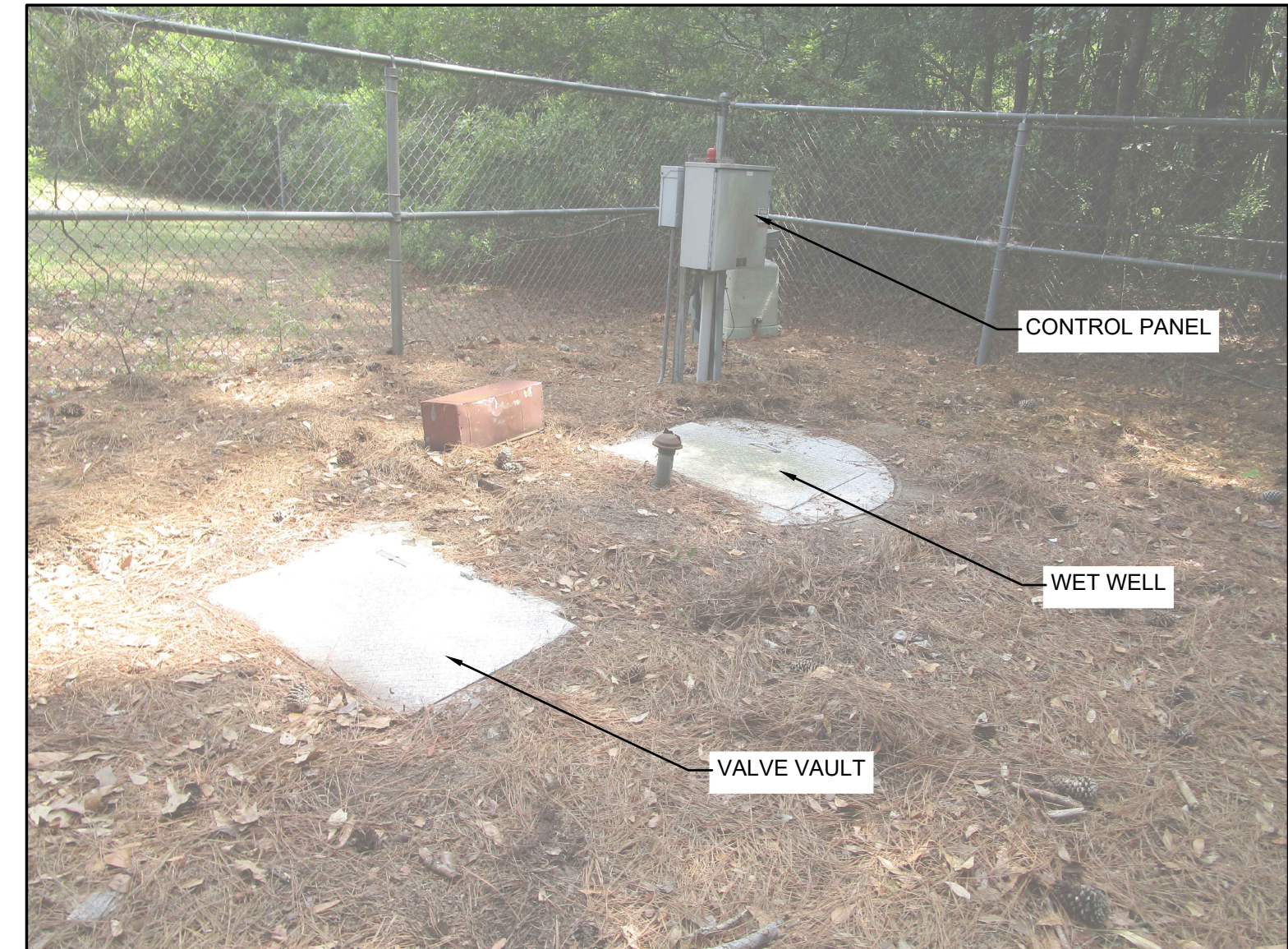
PHOTO-6 LOOKING NORTHEAST AT PUMP STATION
